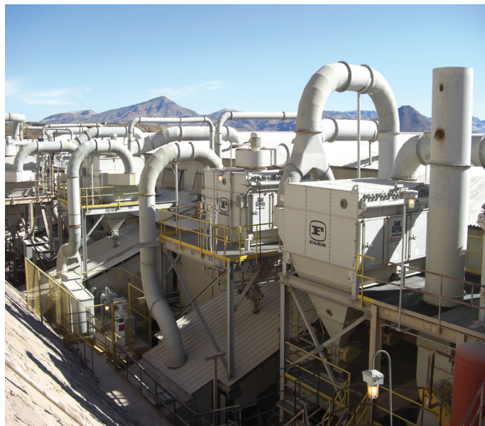
Farr Air Pollution Control system.
