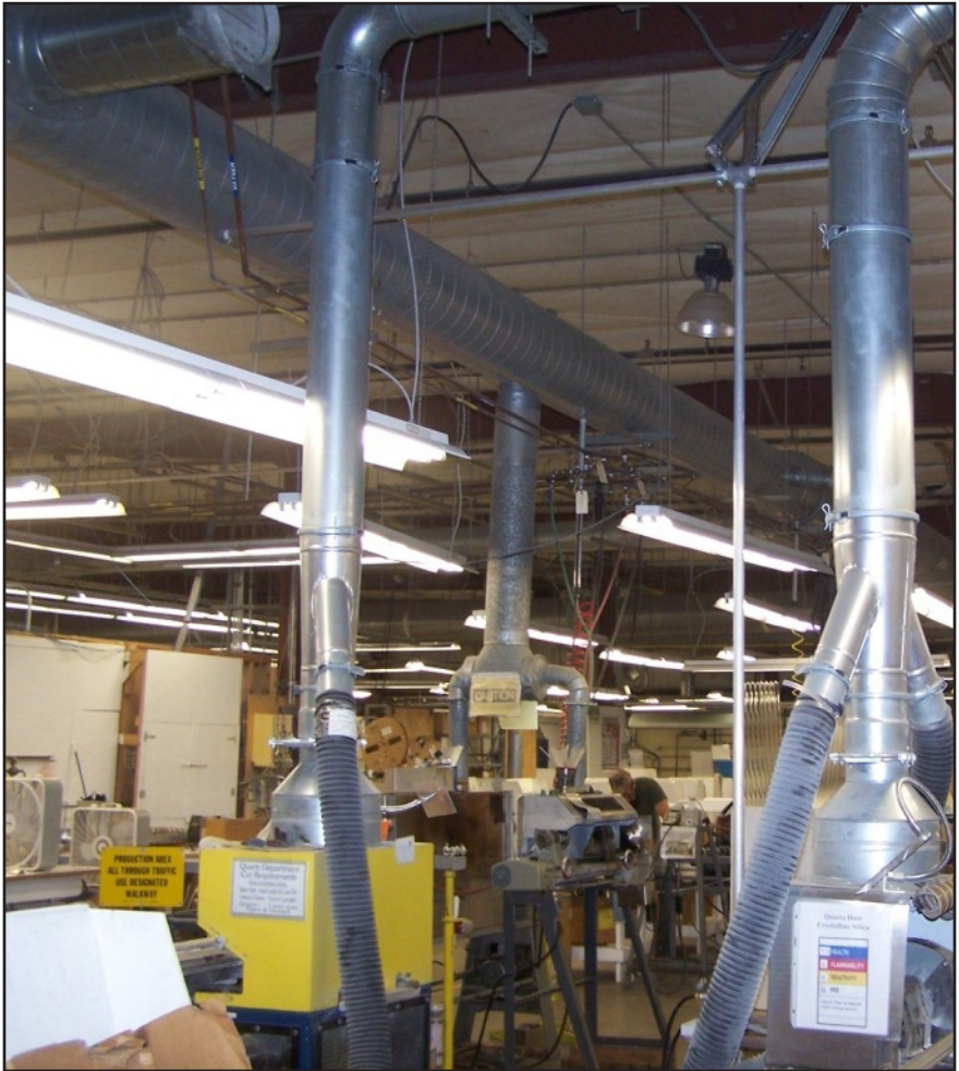
Ducting from the saws inside the building to the Farr dust collector outdoors.
