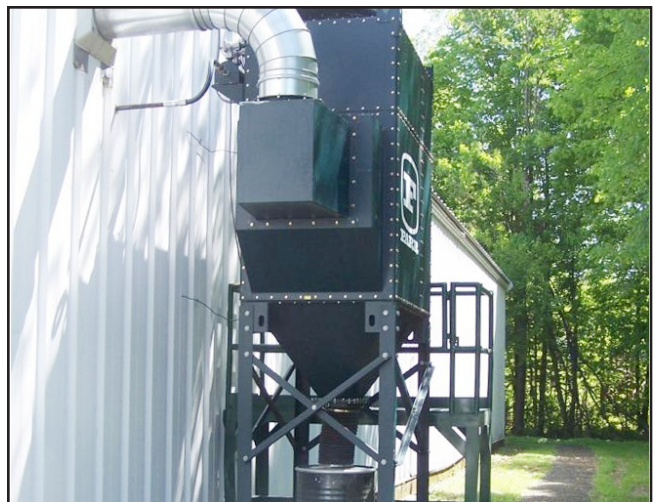
GS6 located on the outside connected to the saws inside the building.
