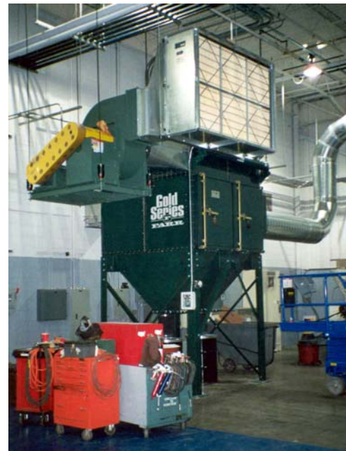
Cartridge collector equipped with safety monitoring filter bank.
