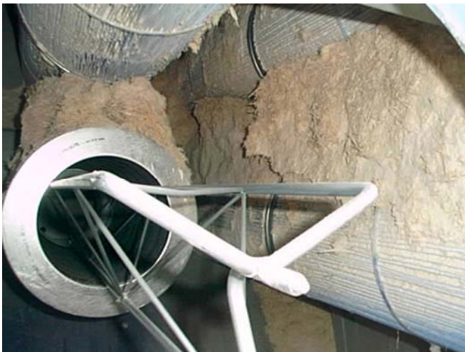
Horizontally mounted filters are subject to uneven dust loading, leading to shorter filter life and potential fire or explosion hazards.
